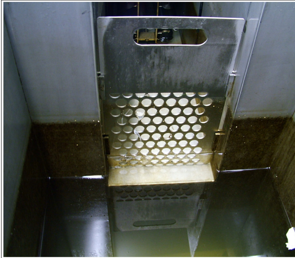
Figure III.4. Baffle Plate at the inlet of the UV channel
